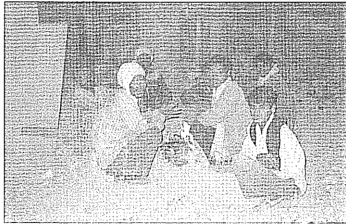
Photo 5. Nighttime Migrant Construction Workers Build an Expansion at SmallCo. Source: Author's Fieldwork, 2003.
